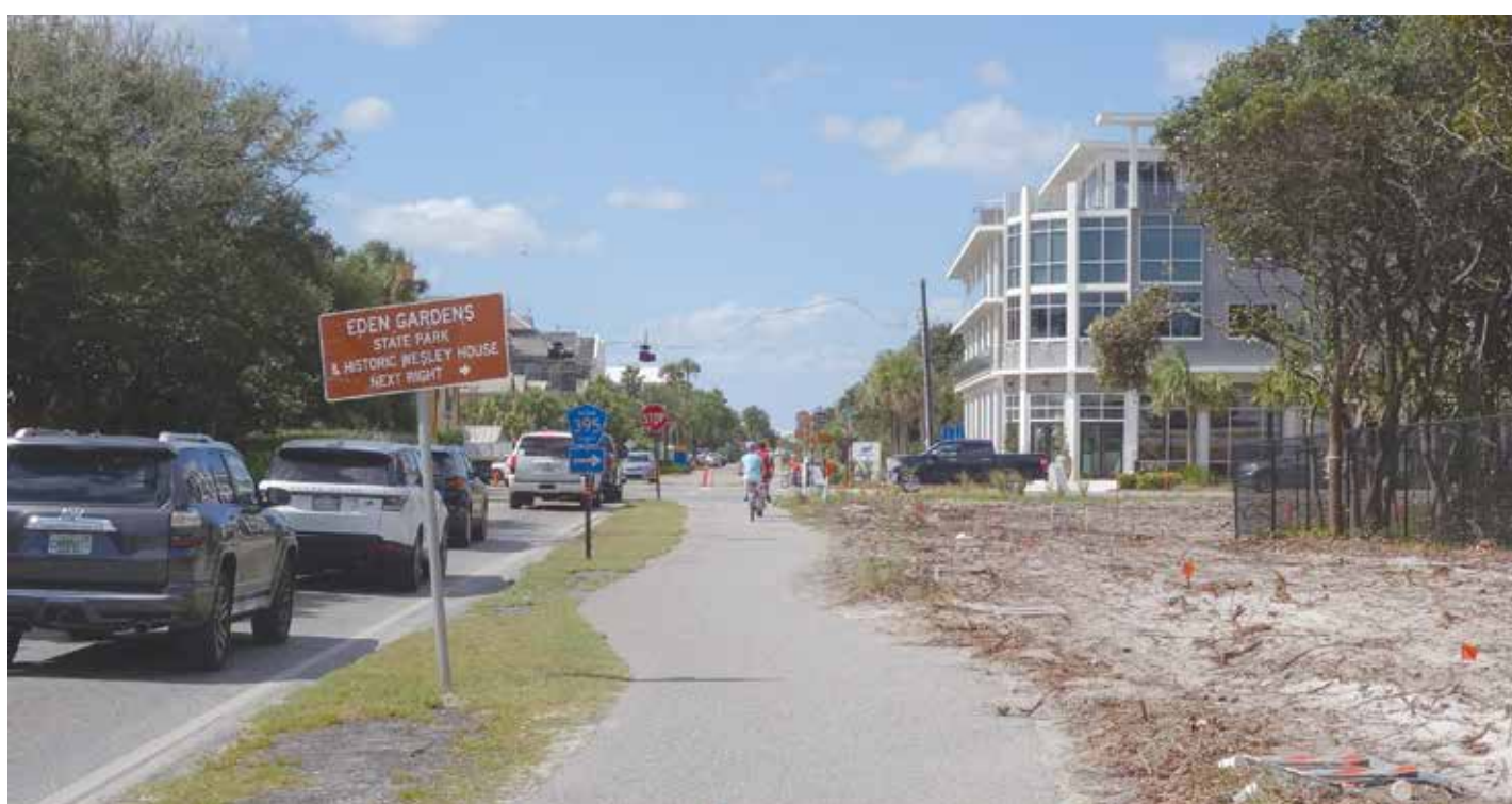
An area northeast of the 30A/395 intersection was recently cleared to begin the construction of turn lanes and the addition of a traffic light. Photo by Mark Schnell
